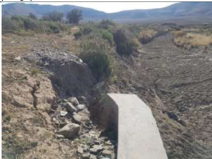
Figure 11: Scouring behind the wall of the big off-take sluice gate, in the background is the riverbed of the Sundays river
