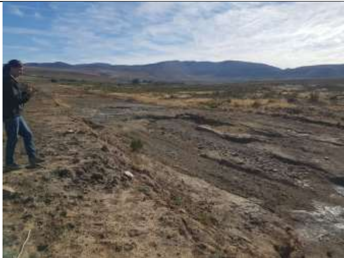
Figure 5: The diversion channel on the right hand side, with the earth berm in the foreground, left
