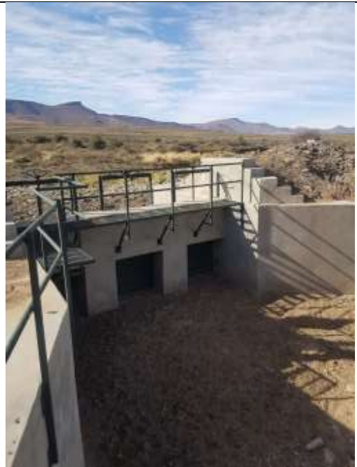
Figure 8: The big off-take sluice gate that diverts water from the Sundays River towards the irrigation basins of Block B
