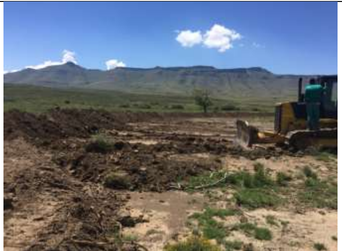
Figure 24: the construction of the dam bays of Block A with a bulldozer
