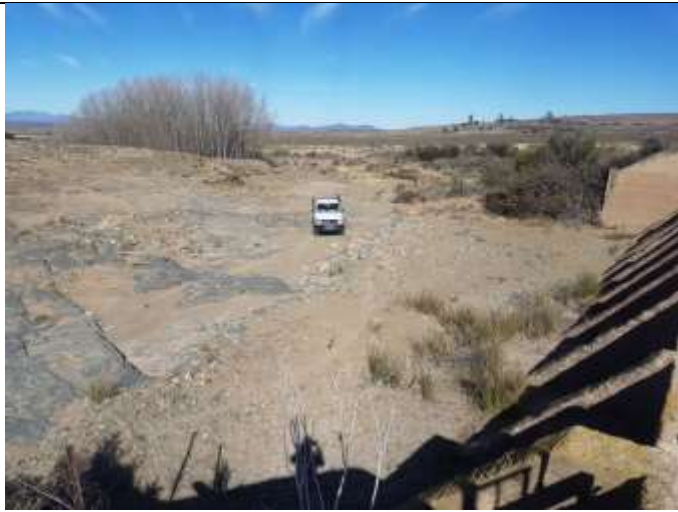
Figure 7: below the spill way, where the water would exit the diversion channel and joins the Sundays River
