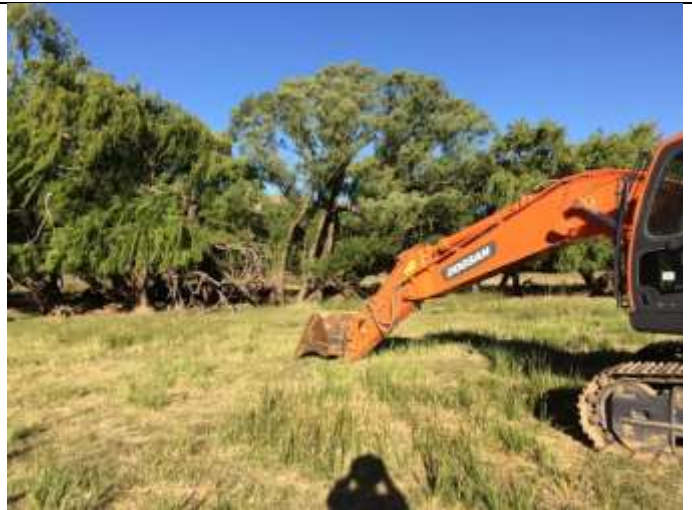
Figure 20: During construction an excavator was used to construct the dam bays and earth berms of Block B
