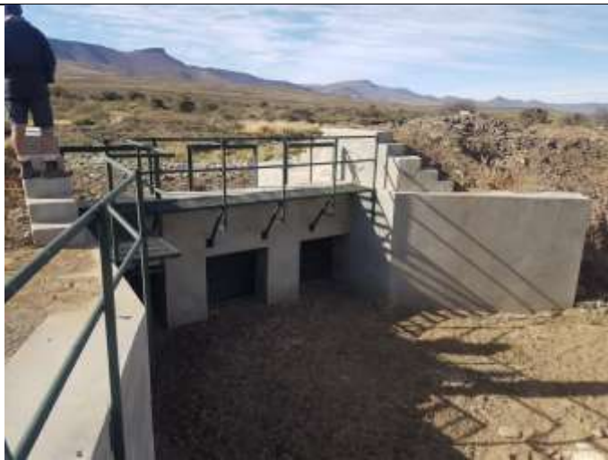
Figure 9: the Big off-take sluice gate, situated north of Block B, photographed from the West
